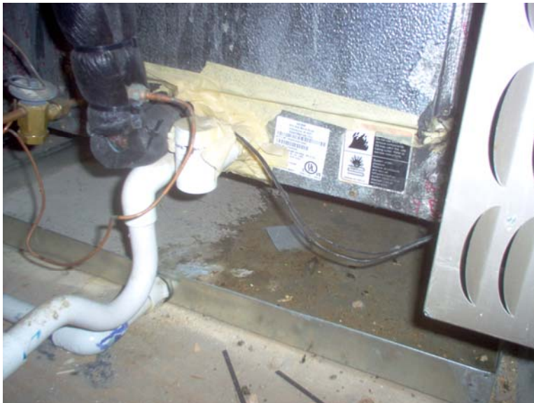
Oil staining at attic mounted HVAC unit.
